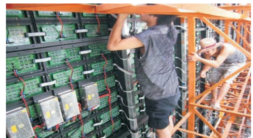
Maintenance is difficult and costly
