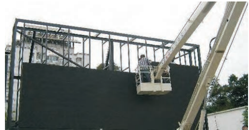
Large, heavy panels are difficult to install and maintain
